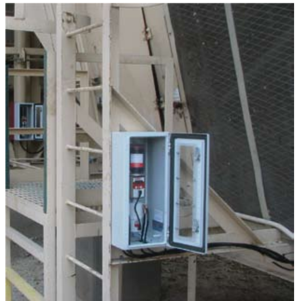
perma PRO MP-6 mounted in enclosure box on gas compression engine cooling fan.
