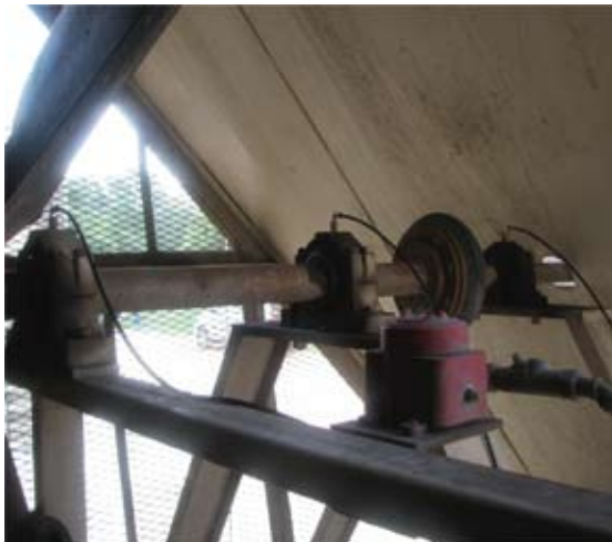
Gas engine compressor fan. Three middle bearings shown with perma 90° tube adapter and 5/16" tubing that is run from externally mounted perma PRO MP-6 automatic lubricators.
