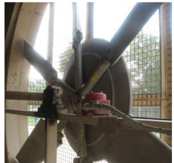
Tubing from PRO MP-6 being run to end bearing on gas compression engine cooling fan.
